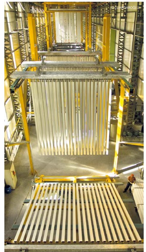
The system installed at ÇUHADAROĞLU remains the only plant in the EMEA region where anodizing and powder coating processes are integrated within the same vertical hybrid surface treatment line for aluminium profiles.
